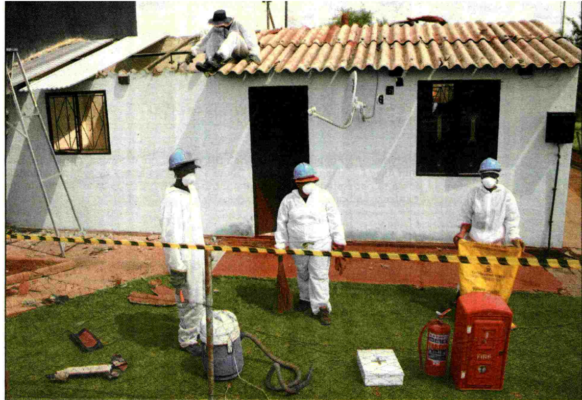
A company replaced asbestos with corrugated iron donated by ArcelorMittal steel company. This was the last out of 1250 houses conducted in Bophelong. Photo: Lazarus Dithagiso
